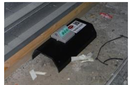
Fig 2: GT sensor mounted on upturned gutter
